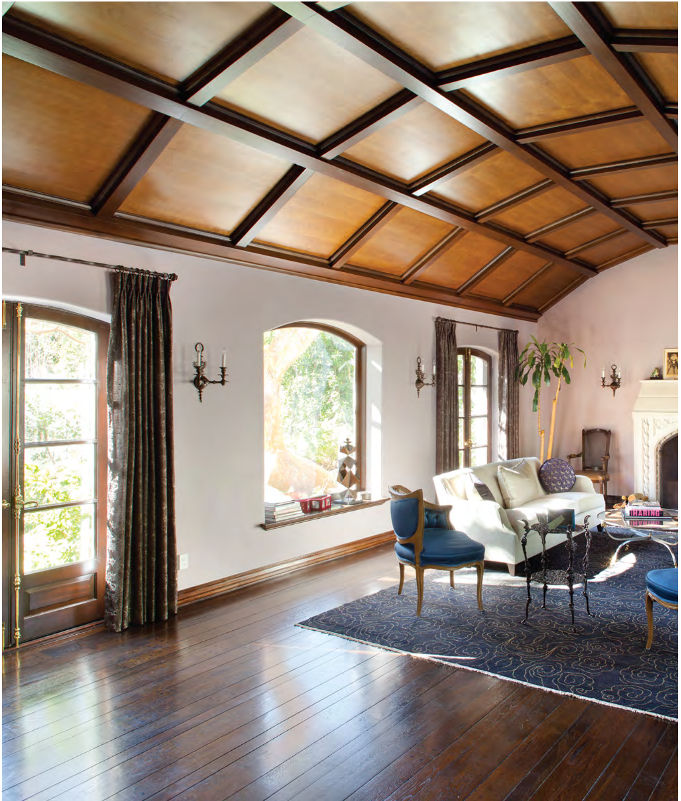
The original barrel vaulted ceiling remained extant despite previous renovations having removed many details
